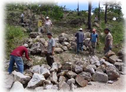
A work group collects large rocks to be used for the foundation of the new tank.
