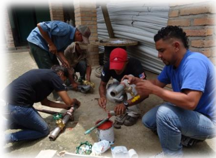
Community plumbers and Water Brigades staff assemble cleaning and control valves to be used in the system.
