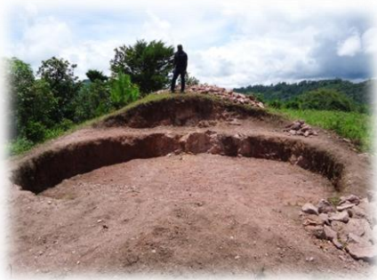
Work groups from Buena Vista leveled the land of the new tank site and dug the area for the tank's foundation.
