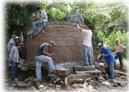
Community members prepare the current tank for repairs by removing the old cement seal.
